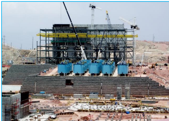
High strength geosynthetics are used to create high walls to support mining facilities and mining substructures.
