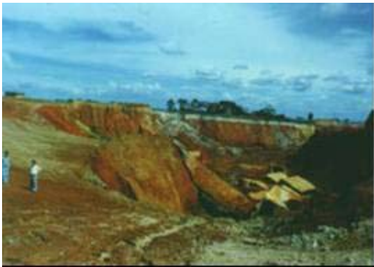
Damages caused by erosion
